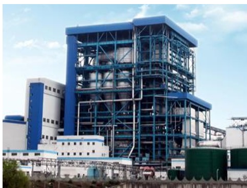
图 2 超临界 600 MW 机组 CFB 锅炉 Fig.2 Picture of a supercritical 660 MW circulating fluidized bed boiler
