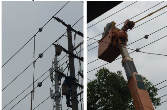
Fig. 4. Photos of dynamic line rating system installation on 35kV and 10kV distribution lines
